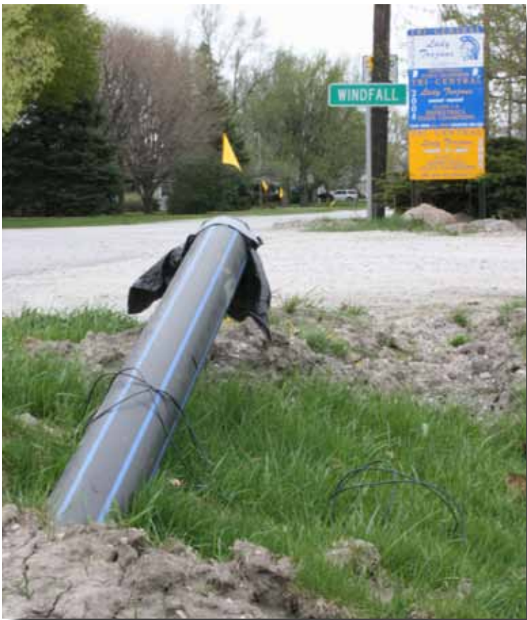
By installing the pipe using horizontal directional drilling, there is no need for open cut, saving the city money.
