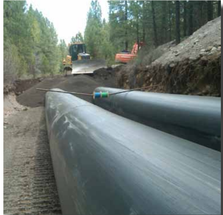
Two 54-inch HDPE pipelines will be buried to convey water from Whychus Creek to a reservoir.
