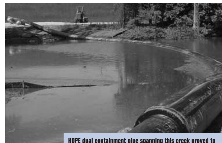
HDPE dual containment pipe spanning this creek proved to be an economical solution for a Midwest energy plant.
