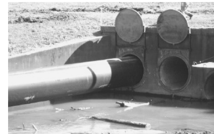
Sliplining with HDPE was a perfect solution to rehab a failing flood control culvert. The project was completed quickly at considerable savings over cutting the floodwall and digging up the existing pipe.
